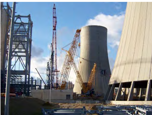
Neurath power plant in Grevenbroich, Germany
