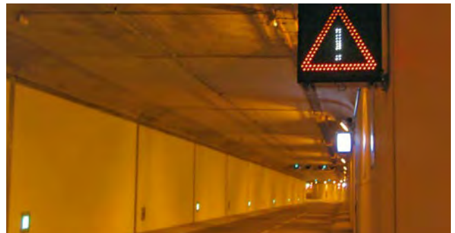
Lighting and signalling systems
