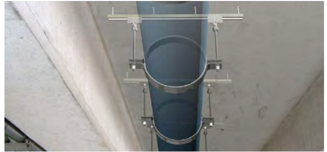
Pipe suspension under bridges
