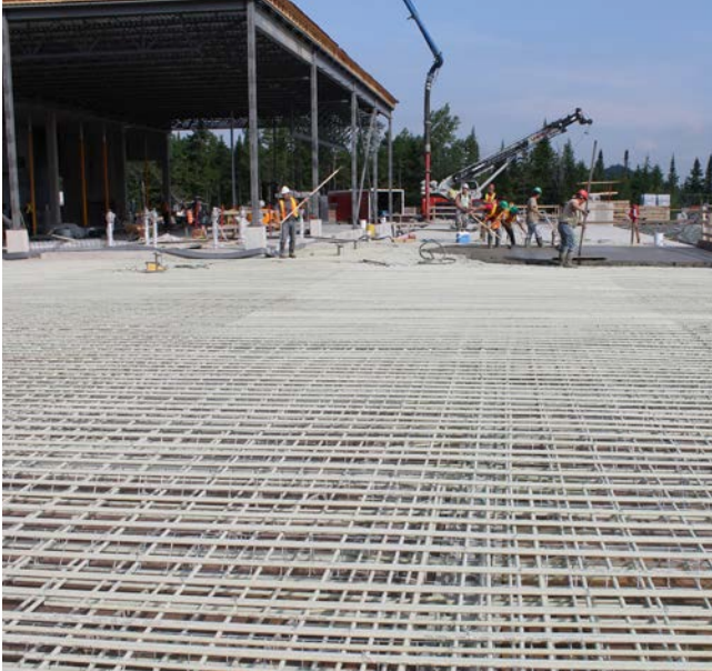
Tanks for sewage treatment plant, floor slab reinforcement Thetford Mines, Québec, Canada
