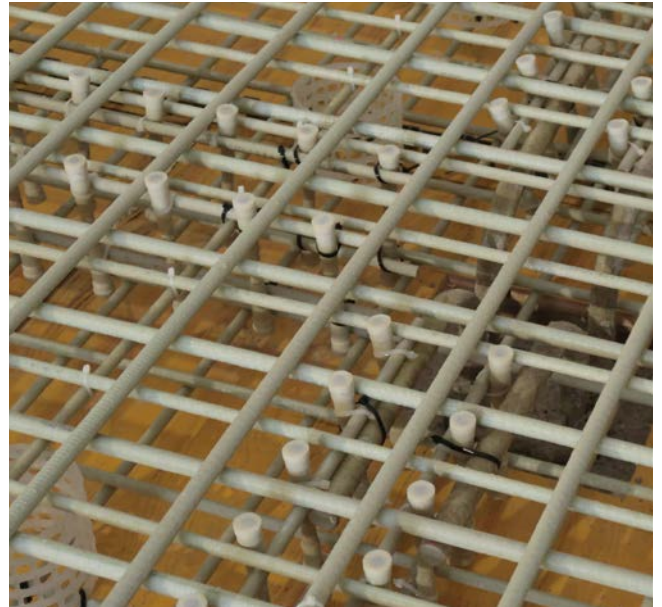
Ground slab and punching shear reinforcement Fusion energy research project Tokamak in Prague, Czech Republic
