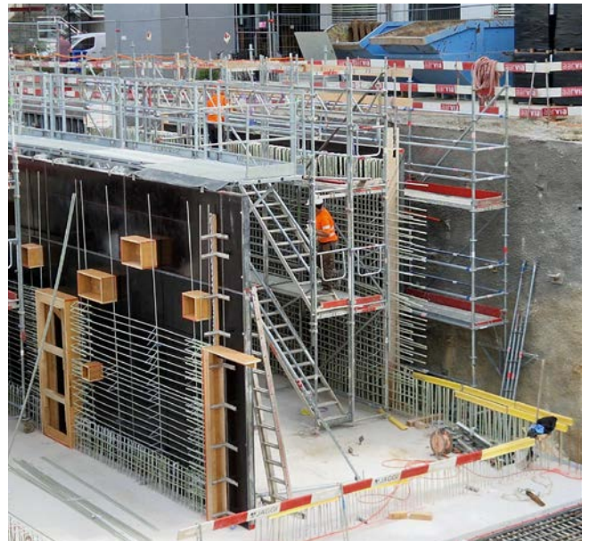
Reinforcement of slab, walls and ceiling of the cryostat-room, Paul Scherrer Institute, Villigen, Switzerland
